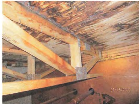
Photo 17: First 3 trusses with water staining
