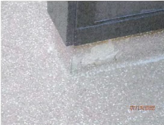
Photo 18: Men's locker flooring damage
