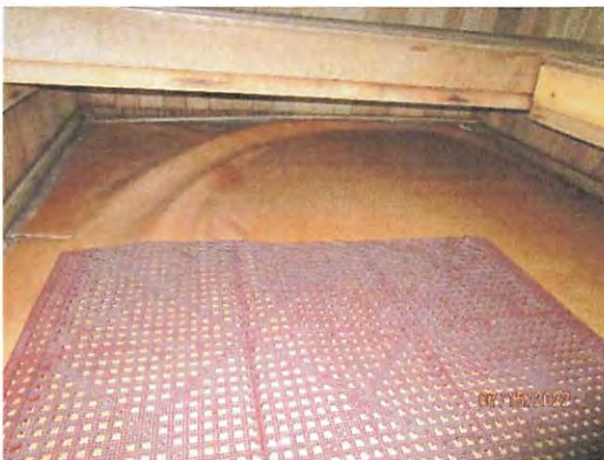
Photo 20: Men's sauna flooring bubbles
