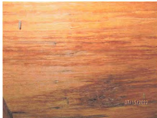
Photo 26: Water staining under men's restroom area
