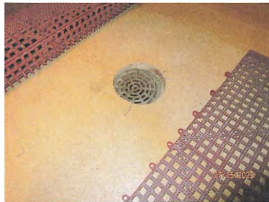
Photo 21: Men's sauna flooring at drain
