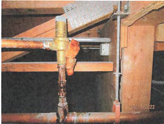
Photo 27: Leaking pressure relief in glycol loop
