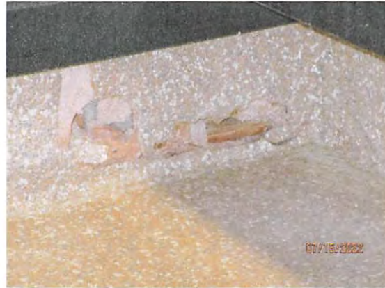
Photo 19: Men's locker flooring damage near sauna
