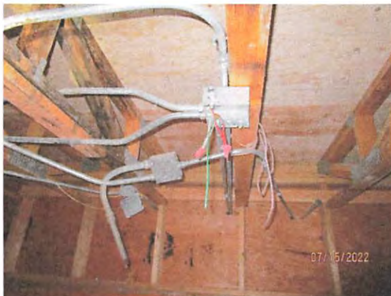
Photo 29: Open junction boxes in crawlspace area
