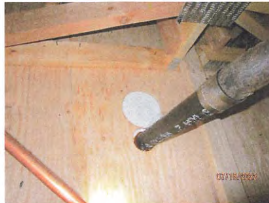
Photo 22: Overcut hole near cleanout.
