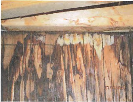
Photo 14: Mold growth on subflooring
