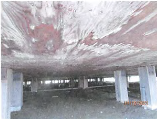
Photo 16: Exterior soffit staining under women's locker area
