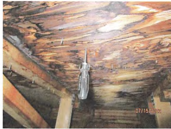
Photo 15: Awl penetration of 3/4" in subflooring
