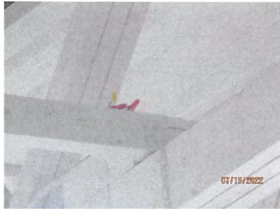
Photo 28: Open junction box in ceiling framing
