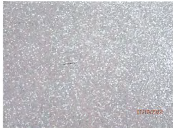
Photo 9: Cracked finish near shower entry
