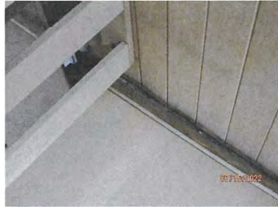
Photo 11: Women's sauna flooring at wall
