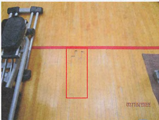
Photo 5: Weight room flooring damage (Note: box outlines damaged area)
