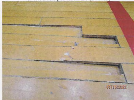
Photo 6: Weight room flooring damage
