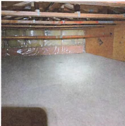
Photo 16. Leak under coupling joint.
