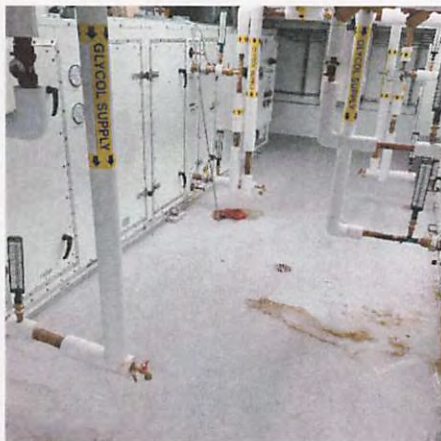
Photo 19. Air heating room.
