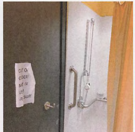
Photo 9. Notice of out of order shower.
