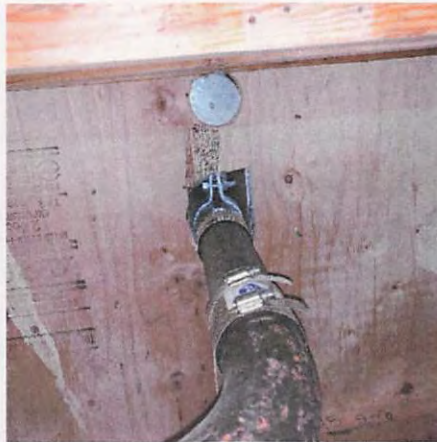
Photo 5. Cutout too large for drain.
