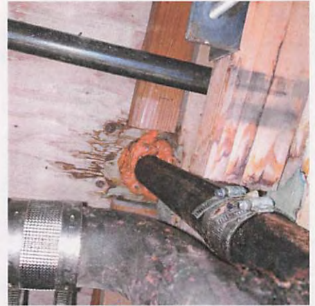
Photo 6. Damage around drain.
