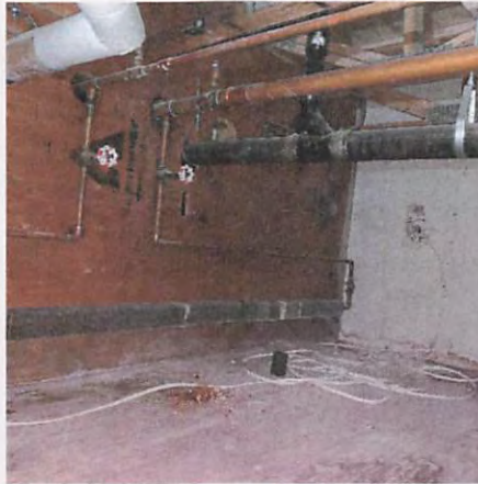
Photo 14. Damage under relief valve.
