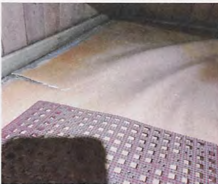
Photo 1. Damage to sauna floor.
