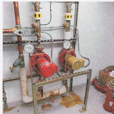
Photo 20. Mechanical room glycol supply loop.
