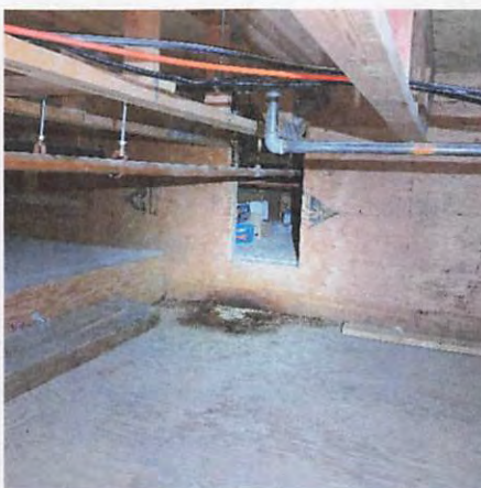
Photo 11. Damage under relief valve.
