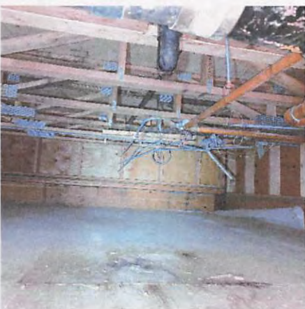
Photo 10. Damage under drain.
