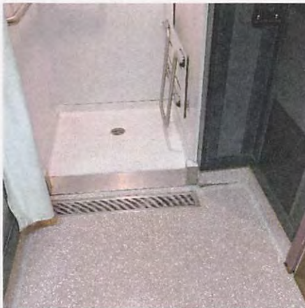
Photo 7. Shower area floor damage.
