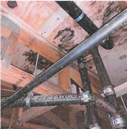
Photo 4. Damage around drains.
