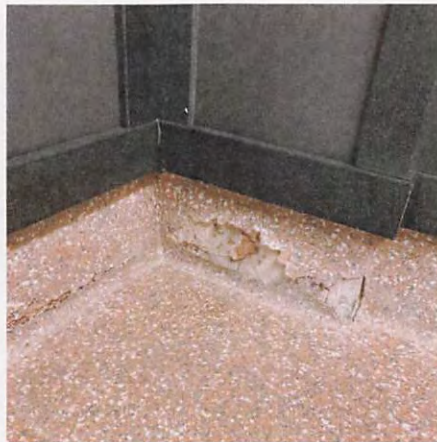
Photo 8. Shower area floor damage.
